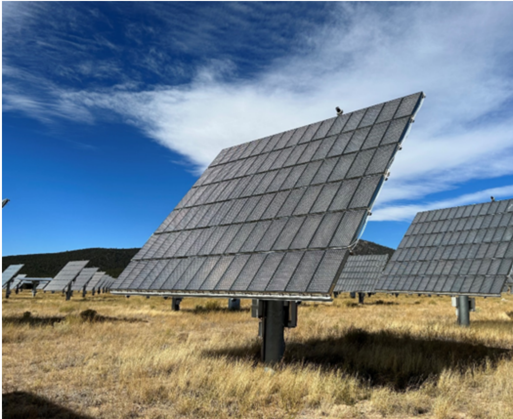
Figure 4-4. Solar installation at Chevron Questa Mine.
